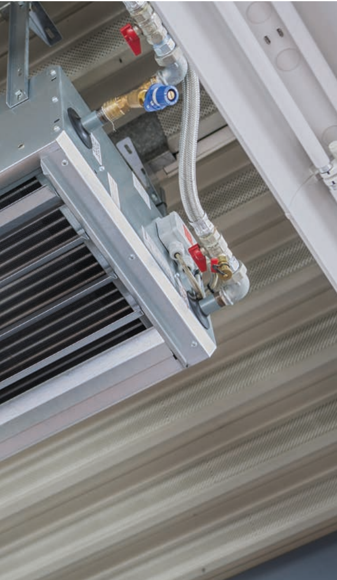
TIP unit heaters installed on the ceiling heat the showrooms belonging to the Seyfarth car dealership in Gotha.
